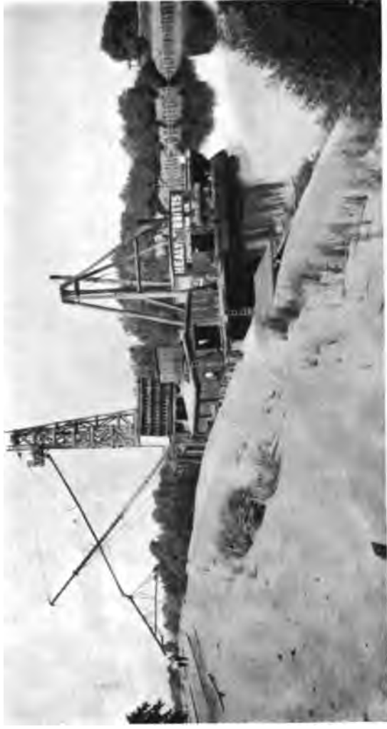
Pouring a concrete road from a barge. This novel method of construction was used along the Sacramento river levee.
